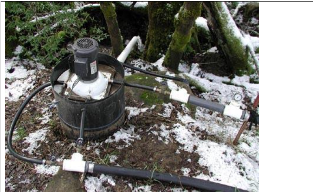
Figure 10. Hydro Power installation. http://www.hipowerhydro.com/Hydro%20Installation%20Pictures.htm
