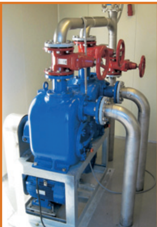
Sewage lift station
