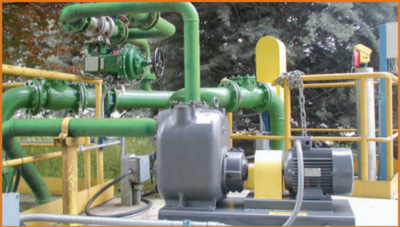
Waste water treatment in a sugar refinery
