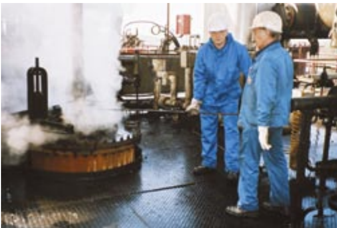
Short Tool in service, during switching mode.
