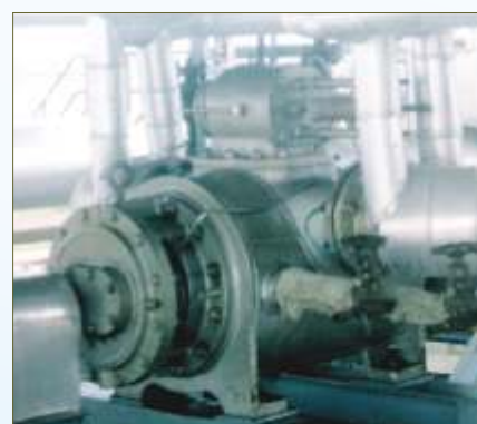
Pumping Bitumen at a facility in Tehran, Iran
