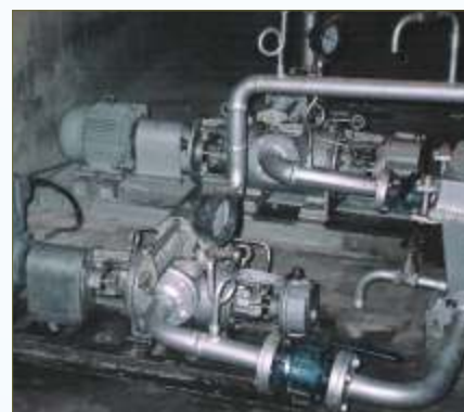
Pumping resins at a facility in Kolkata, India
