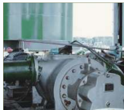
Pumping Molasses at a facility in Vietnam
