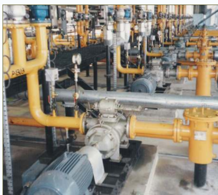
Pumping Lube Oil at Lube Oil Blending Plant in Haldia, India
