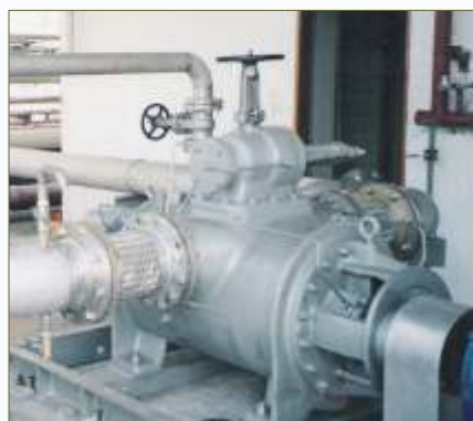
Pumping Chemical at a facility in Malaysia
