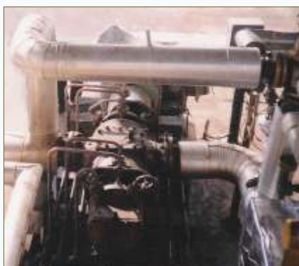
Pumping Black Liquor at a facility in Turkmanistan
