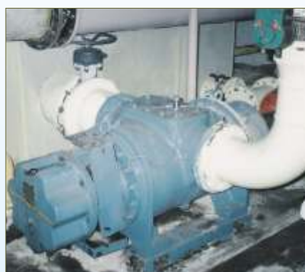
Pumping Viscose at a facility in Indonesia
