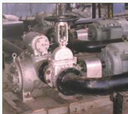
Pumping Crude Palm Oil at a facility in Haldia, India
