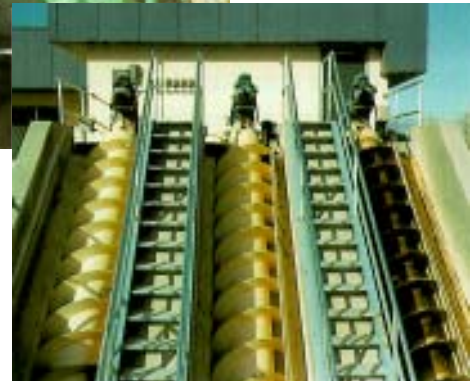
The screw pumps gentle spiral lift reduces break up of floc when handling return activated sludge.
