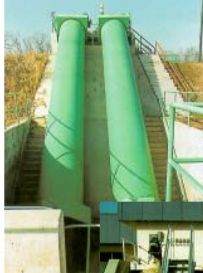
Screw pumps are non-clogging so they can handle most objects in raw wastewater influent.
