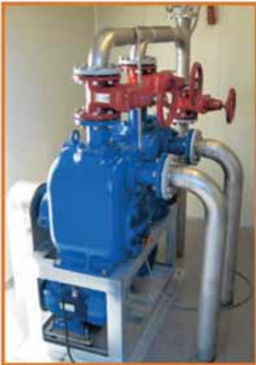
Sewage lift station
