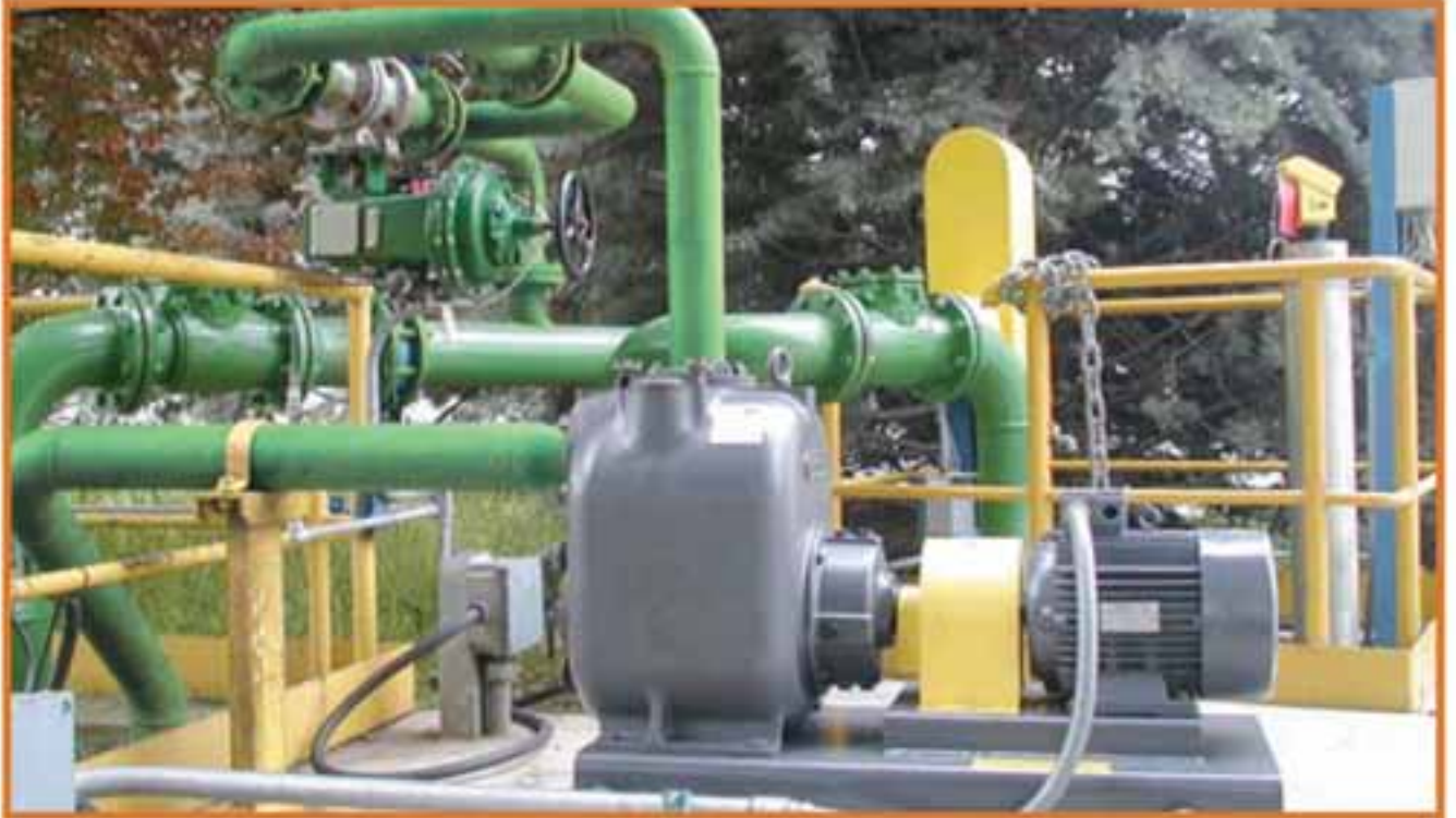
Waste water treatment in a sugar refinery
