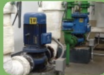
In line Circulation Pumps
