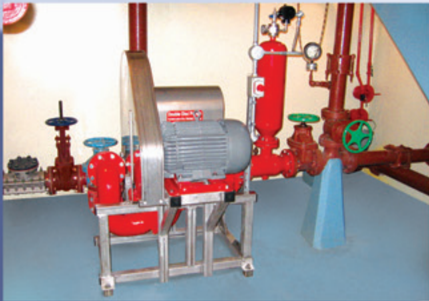
City of Warminster, PA WWTP
