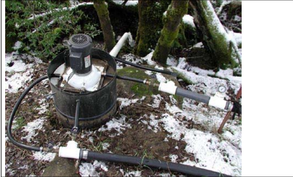
Figure 10. Hydro Power installation. http://www.hipowerhydro.com/Hydro%20Installation%20Pictures.htm
